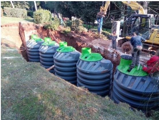
Picture 5: Installed tanks in a row
