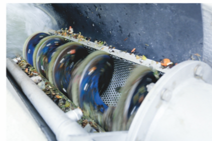
Mechanically cleaned screens
