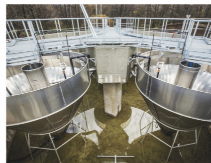
Inserted settling tanks
