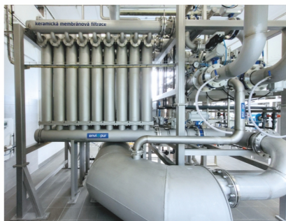
Bolevec Pond WTP (CZ)
